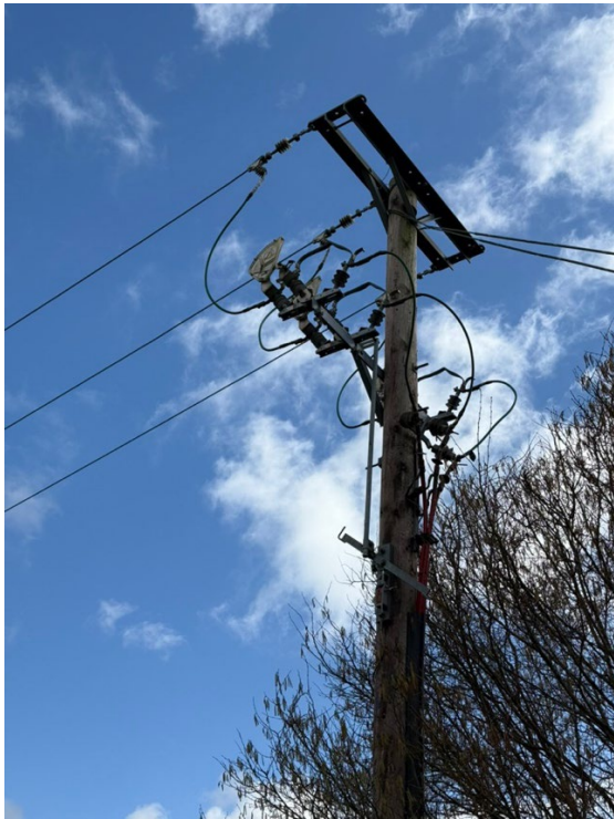
Figure 2 UKPN Pole 810603 with isolator switching
